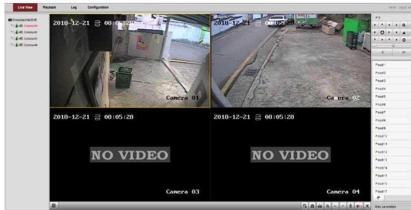
Fig.3. Access and control of the CCTV system
